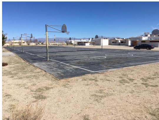
MJH58 – West Play Field (basketball/tetherball) pulverize asphalt court at west end of campus; remove goal posts & tether ball poles; bf/compact; import clean fill dirt; smooth finish grade; no ponding
