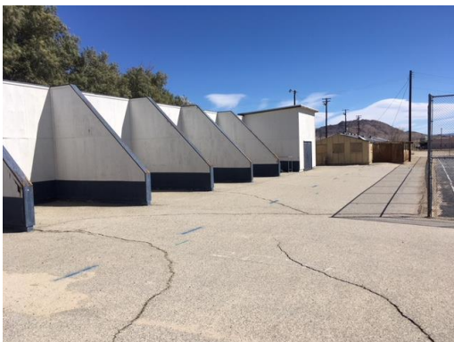
MJH50 – saw cut asphalt pavement adjacent to C.L. fence at basketball court; pulverize asphalt
