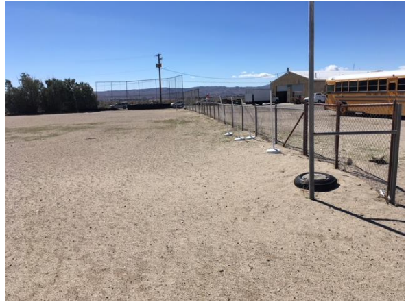
MJH55 – remove softball field line fence, posts, bf/compact; import clean fill dirt, smooth finish grade entire softball field east; no ponding in finish grade
