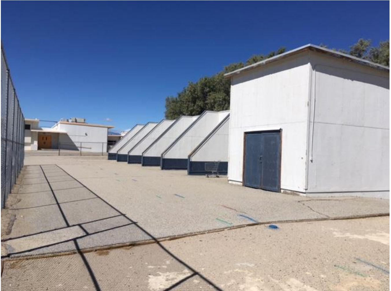
MJH 50 & MJH53 – demolish ball wall, building, stem wall & concrete footing, bf/compact; saw cut existing asphalt pavement adjacent to C.L. fence at basketball court; pulverized asphalt and smooth finish grade; import clean fill dirt as needed for smooth finish grade where MJH 50, MJH52, MJH53, MJH54, MJH55 & MJH56; no ponding in finish grade
